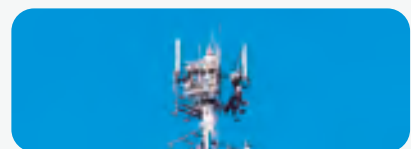
5G wireless infrastructure
